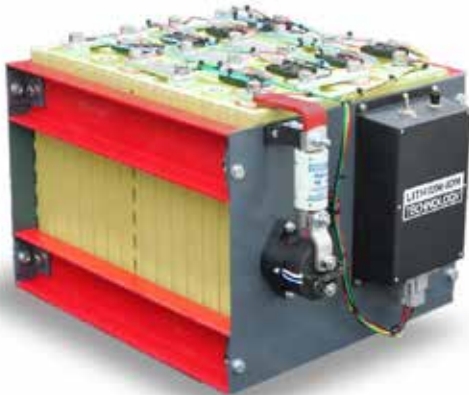
TOP: GBS lithium-ion battery bank intended for an RV. PHOTO COURTESY STARLIGHT SOLAR
